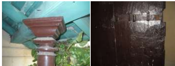
Fig 8. Wooden columns(Rosewood) as seen in courtyard. The latch which is still intact from the day of construction
